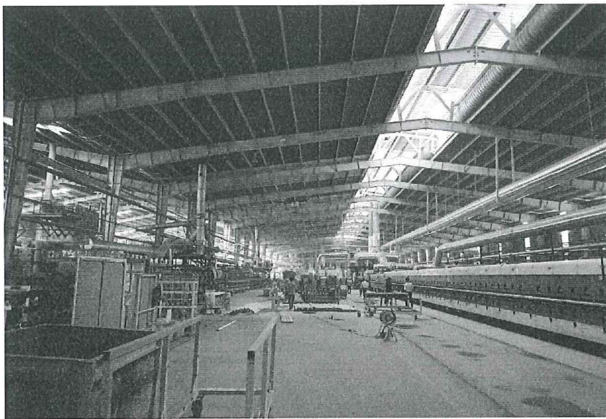
Continuous Tile kiln system and heat recovery pipeline
